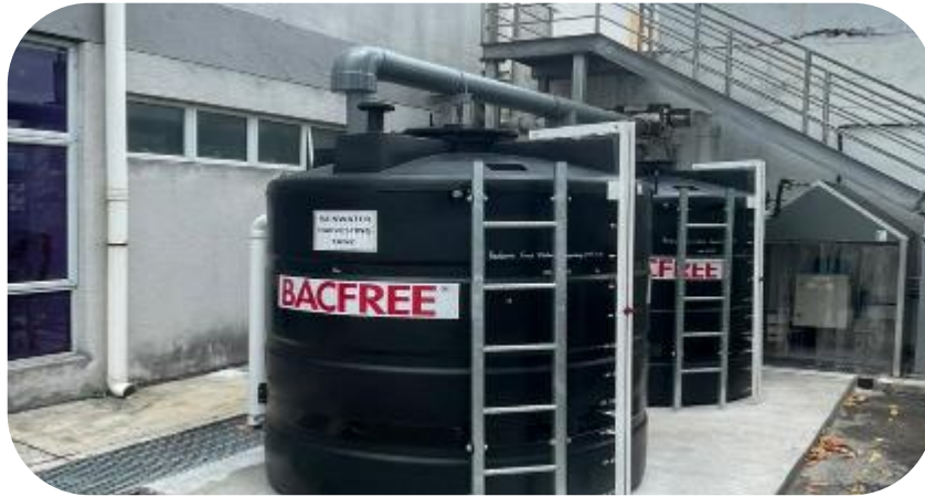
Rainwater Harvesting at AHSB
