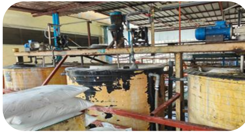
Reuse treated water for dilution at WWTP at OMI Shah Alam
