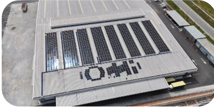
336 kWp Solar Panel at OMI Sg Choh
