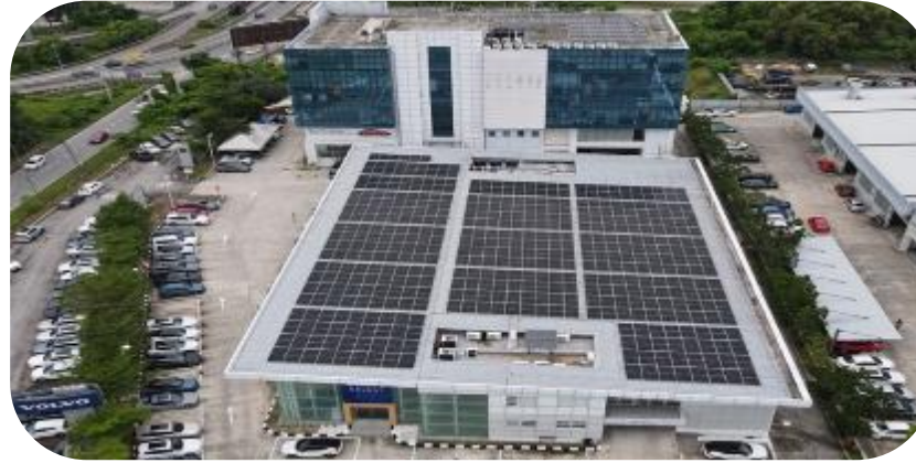
314 kWp Solar Panel at FAHB Glenmarie
